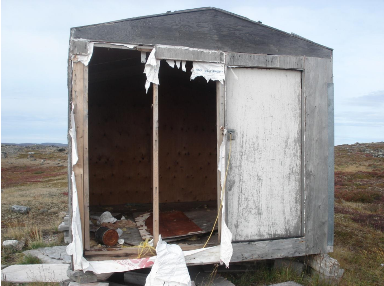
Figure 3: A cabin damaged by a grizzly bear. Source: anonymous Baker Lake participant
